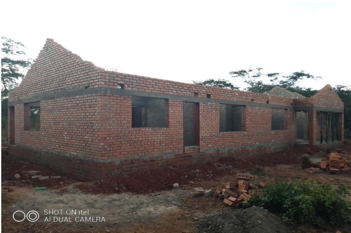
This is the structure that was completed in May 2021 but has remained at the same level since then
